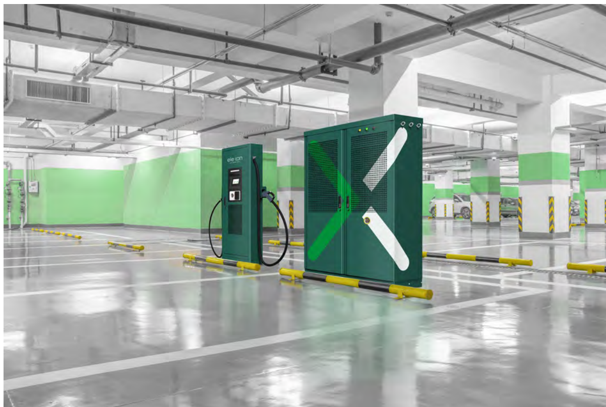
Image 3: The new AC charging station from elexon offers up to 3 terminals with 2 charging points each and a PowerBank as a base.
